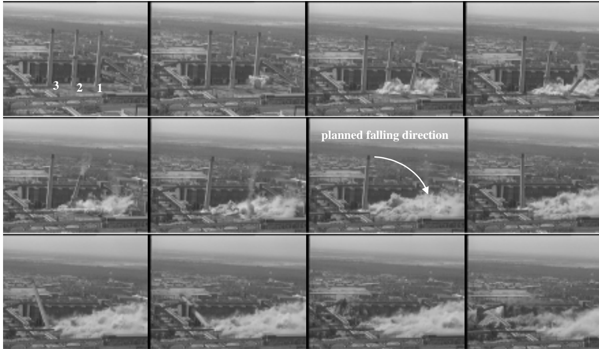
Fig. 1: Unsuccessfully controlled chimney demolition, Spremberg Germany, 10th July 1999; the third chimney was planned to fall to the right direction, but fell instead over the building.
